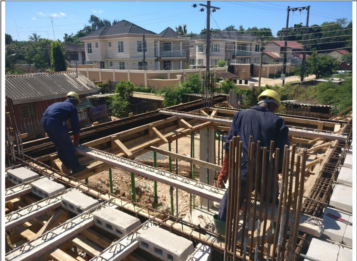
Photo 4: Upon receipt of both ends, the two personnel moves the joists to its predetermined positioned established with chalk marking on the sides of formwork of main beams.
