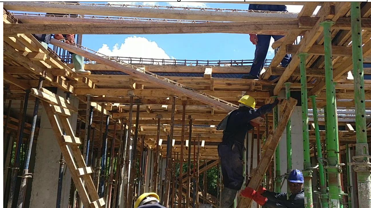
Photo 3: The climber make use of the second ladder to deliver the second end of the joist. At this stage ladder stability is of paramount.
