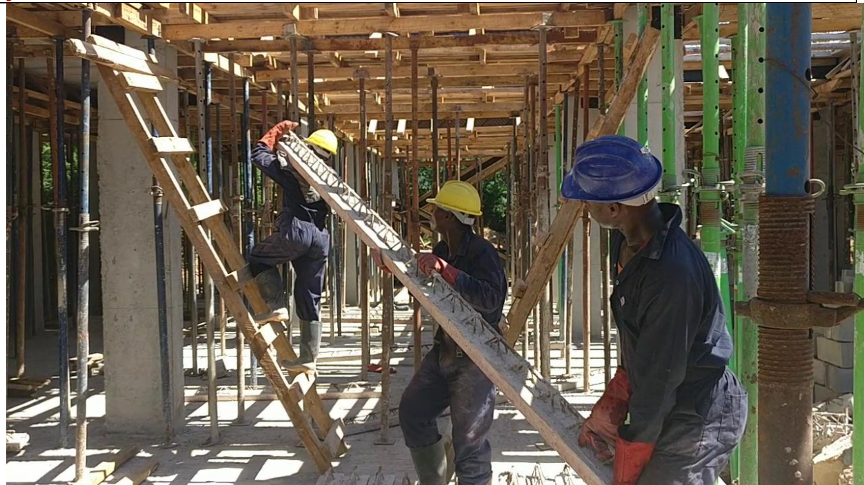
Photo 1: Three personnel handles lattice joists with the climber carefully climbing up the ladder.
