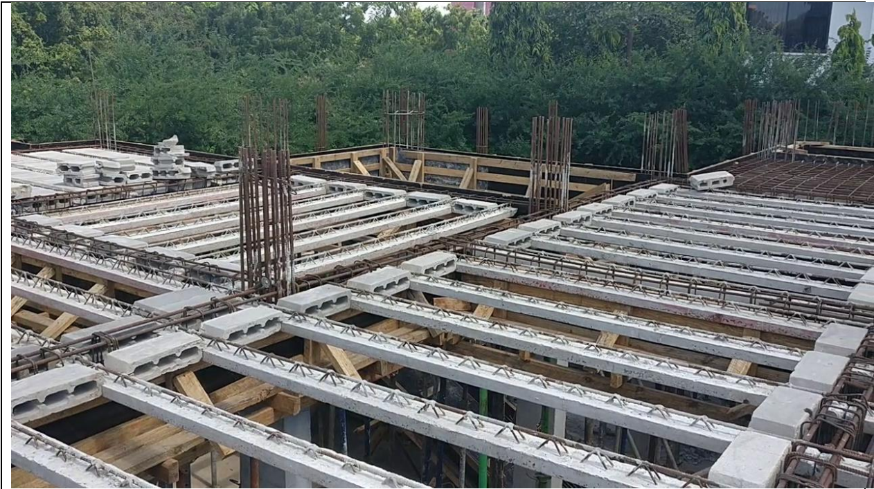
Photo 6: Start up filler blocks positioned on both ends to ensure uniformity upon completion
