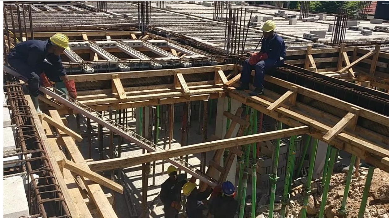
Photo 2: Two personnel receives lattice joists to be supported on main/primary beams, one end of the joist has been received, the other was temporarily supported on the second ladder before the climber could get it to the other personnel.
